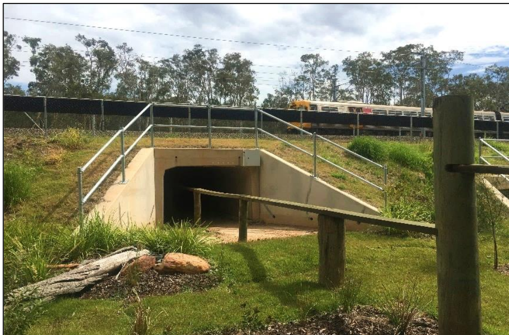
Plate 1: A culvert for Koala crossing below a railway line showing crossing furniture and fencing (source DES 2022).
